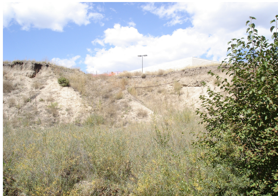
Exhibit IV-11: Bank Erosion near Commercial Development
