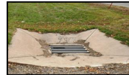
CDOT Type C Inlet in Depression
