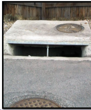
Denver No. 14 Curb Opening
