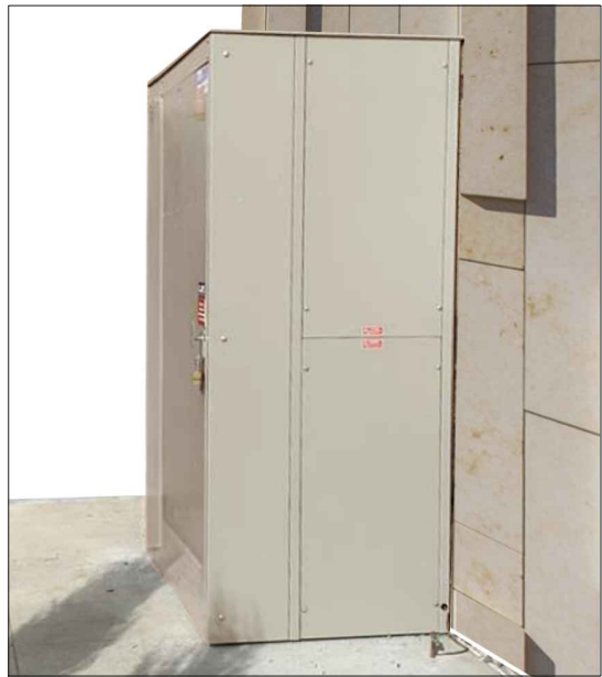
8 Painted Euserc Cabinet
