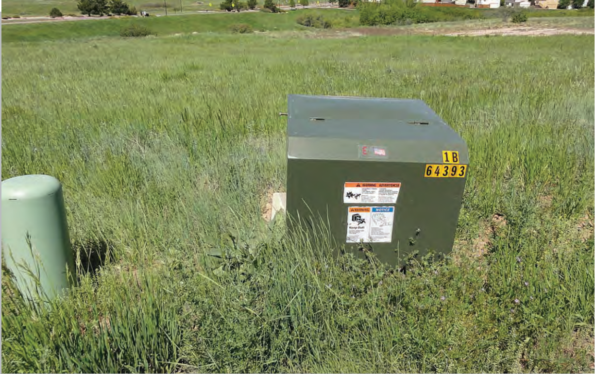
Photo 3 - View of a pad mounted transformer near the southeast corner of the property.
