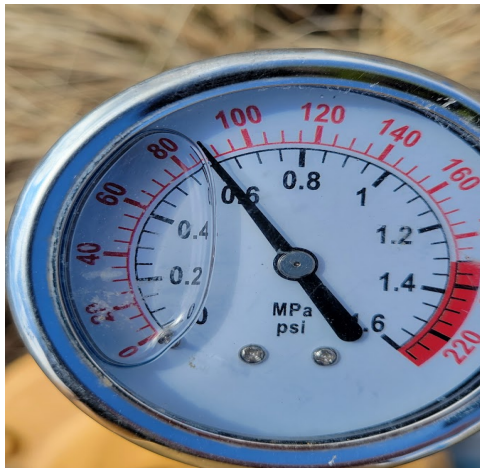
Residual Pressure -87 PSI
