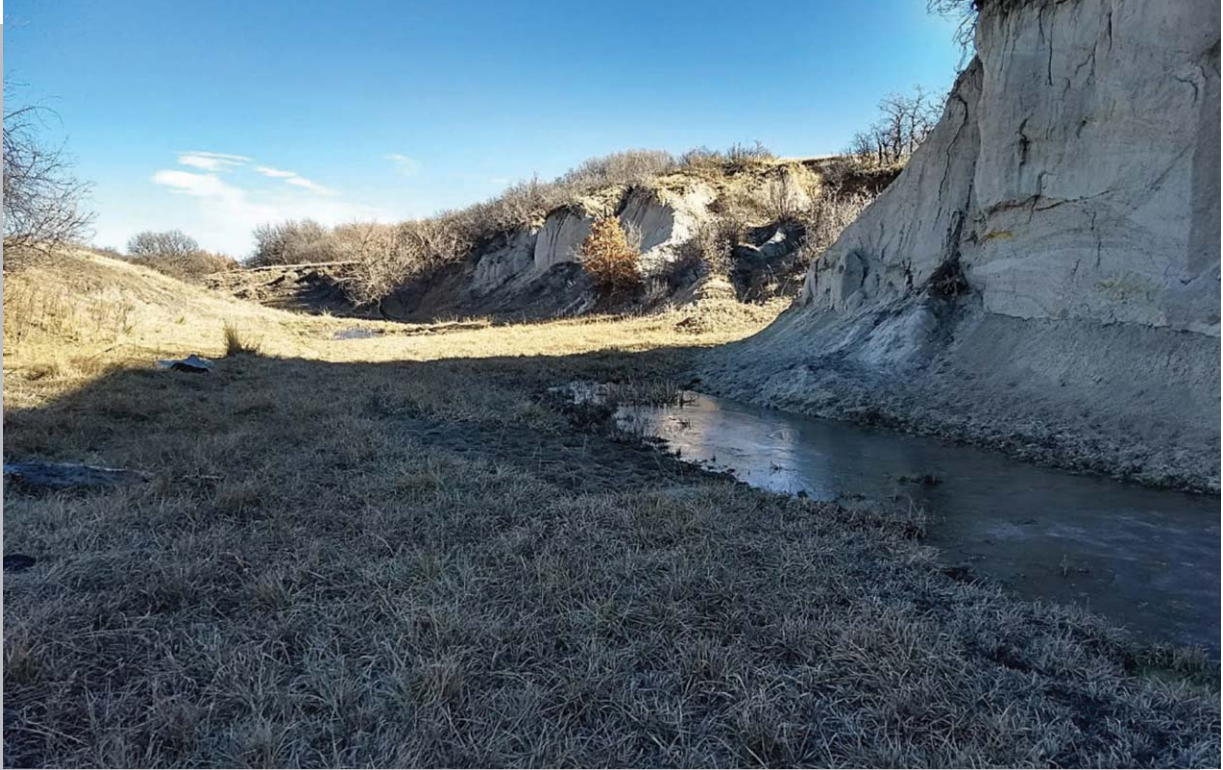
Photo 1 - View of extreme channel degradation on Scott Gulch following the 2013 floods. View is to the northeast..
