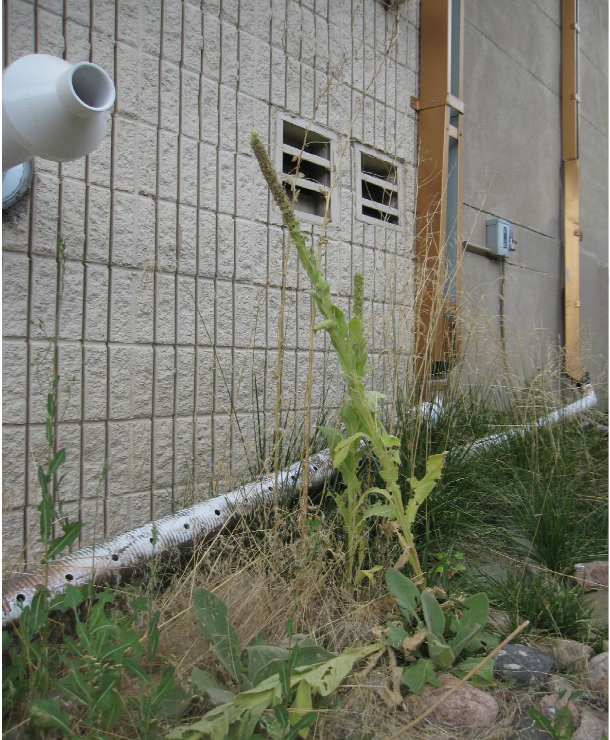
Photo 4. Note the presence of dried cheat grass along with other weeds and grasses below the vents. The rock border will be ineffective in preventing flames from reaching the building.
