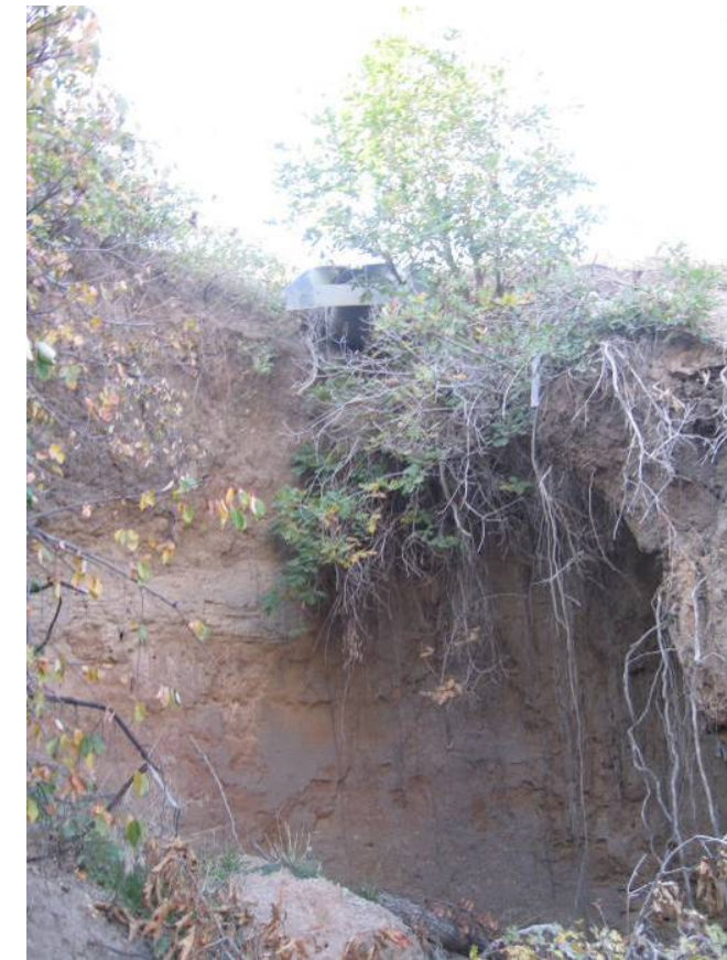
Undercut Culvert on Industrial Reach 1
