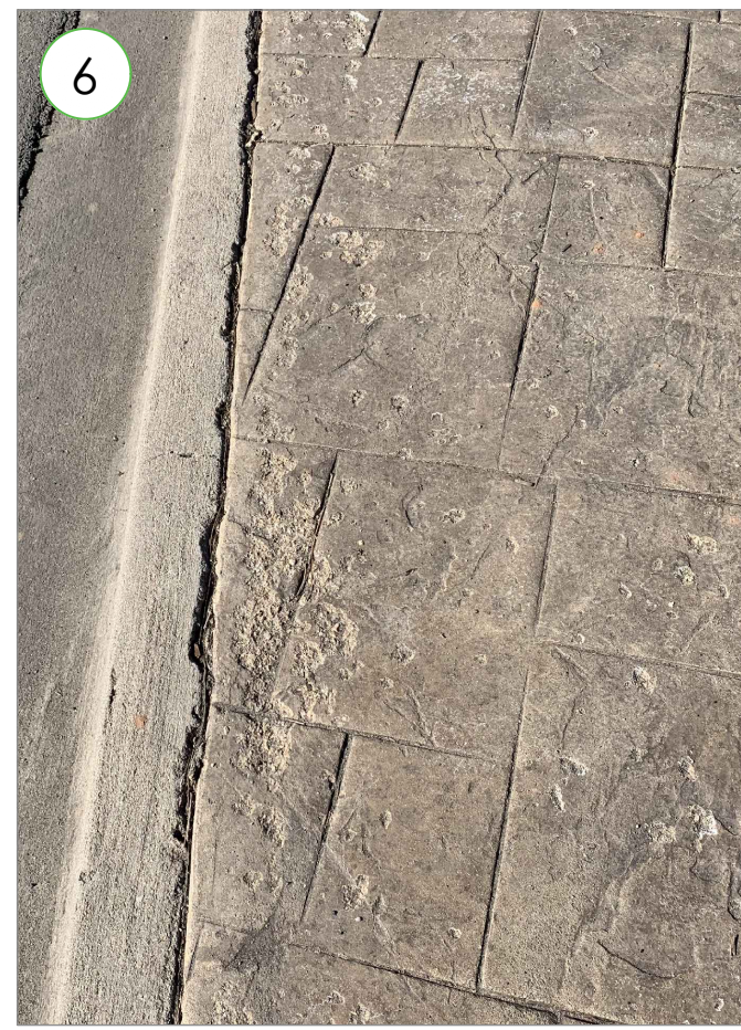
VIEW LOOKING AT FLECKING/ SPALDING OF EXISTING STAMPED/COLORED CONCRETE.
