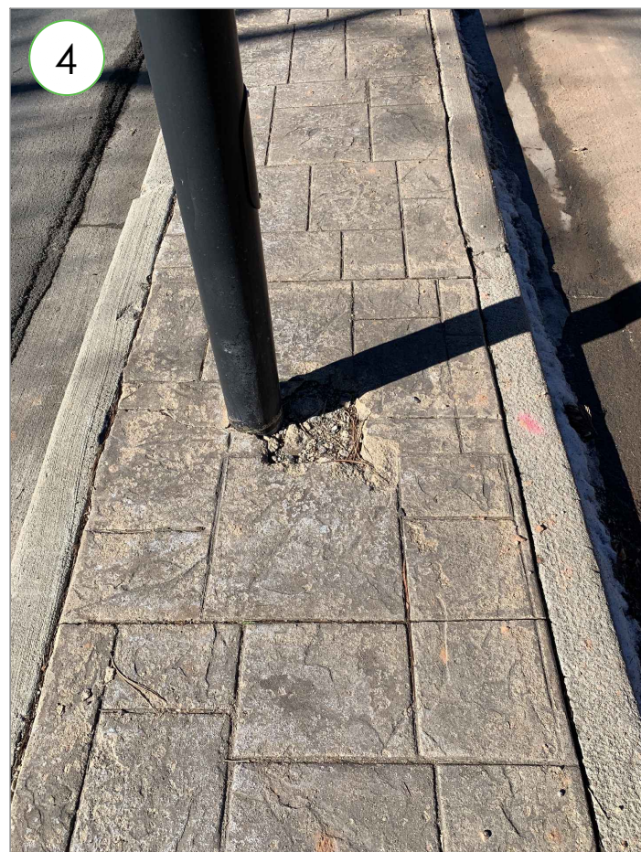
VIEW LOOKING AT EXISTING STAMPED/COLORED CONCRETE AND DAMAGE AT THE BASE OF LIGHT POLE.
