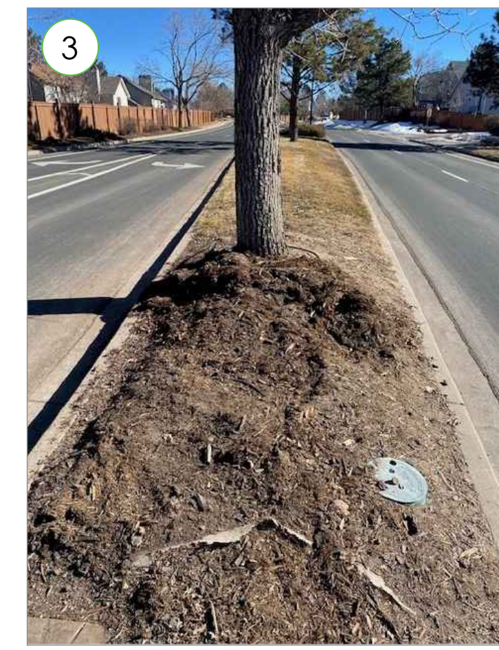
VIEW LOOKING EAST TOWARDS EXCESS MULCH AND SOIL.
