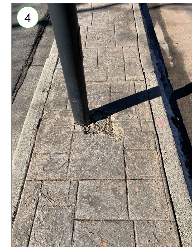
VIEW LOOKING AT EXISTING STAMPED/COLORED CONCRETE AND DAMAGE AT THE BASE OF LIGHT POLE.
