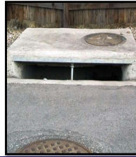
Denver No. 14 Curb Opening
