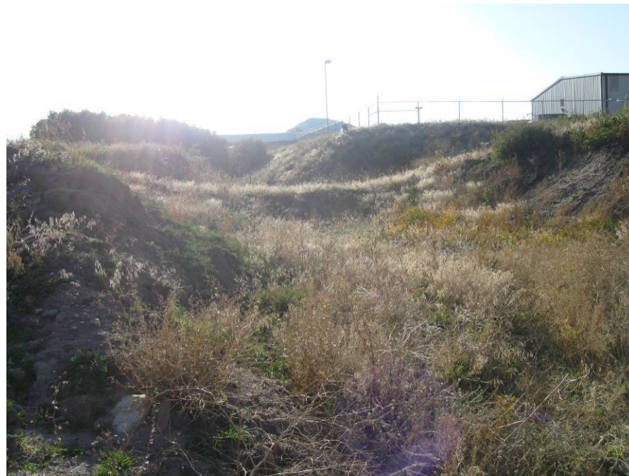
Eroded Channel in Reach 2 of the Industrial Channel
